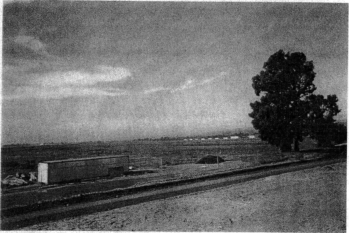
Photo 11. Project area, facing northwest. Highway 84 is under construction east of the site. The project area only includes the grassland beyond the construction site.
